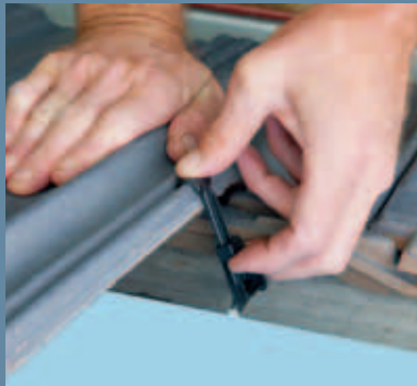
Swivel clip into position over tile and press firmly down to water course of tile
